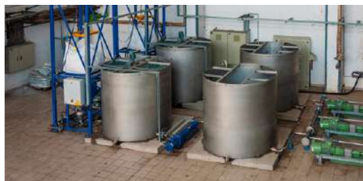
Level monitoring by triggering an acoustic or visual device
