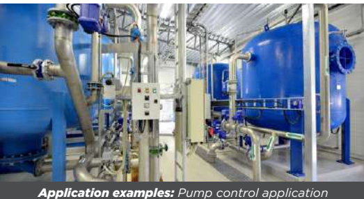
Application examples: Pump control application
