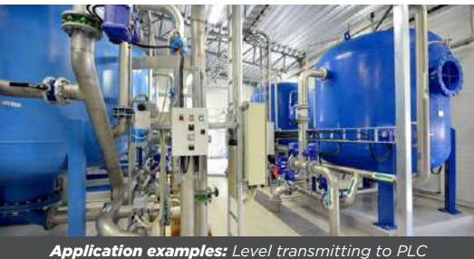
Application examples: Level transmitting to PLC
