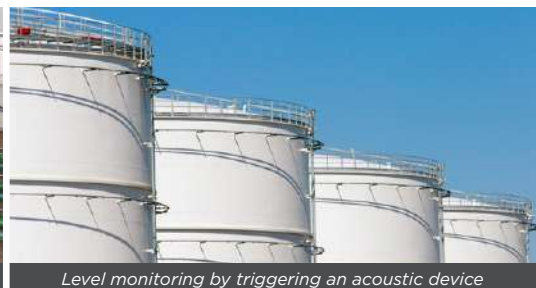
Level monitoring by triggering an acoustic device
