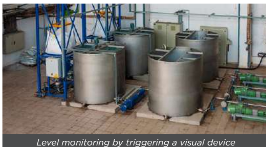
Level monitoring by triggering a visual device
